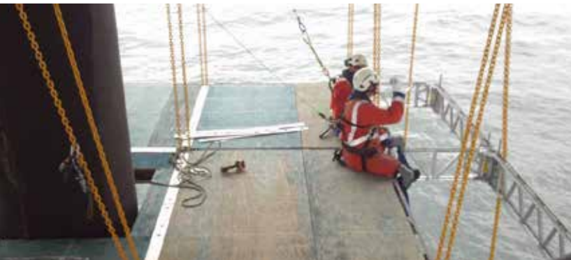
BrandSafway sent trainers to New Zealand to work with the on-site installation team.
