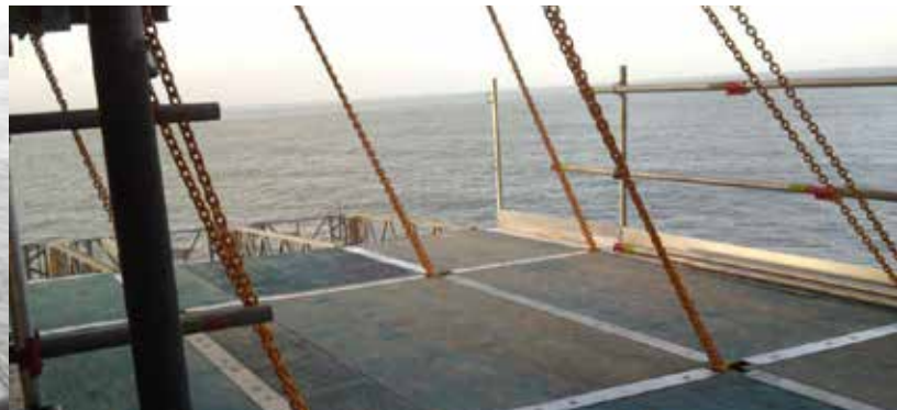
QuikDeck delivered a safe, smooth surface to paint the entire offshore natural gas platform.
