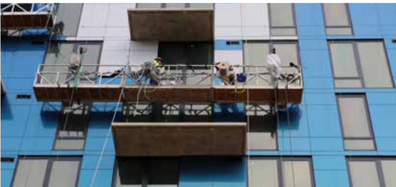
Skilled trades that used the swing stage platform also included those installing window caulking. ⤴
