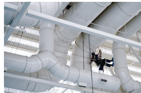
Rope access reduces schedules and costs on at-height work — from fireproofing and refractory to insulation and coatings.
